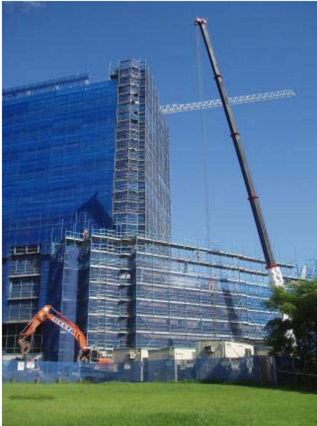
Above: The Sturt House demolition in progress, with the R&E Building in the background.
